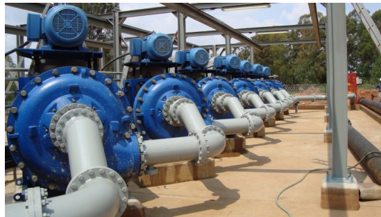
Heavy pumping system for tailing slurry
