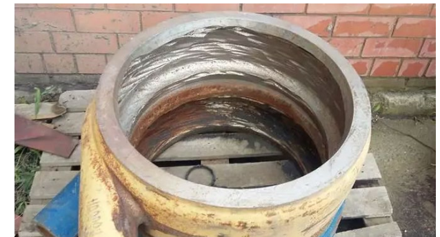
High erosion inside the pumps
